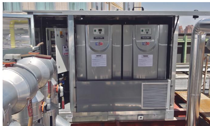
Foto: Adisa Heating (Hitecsa)
